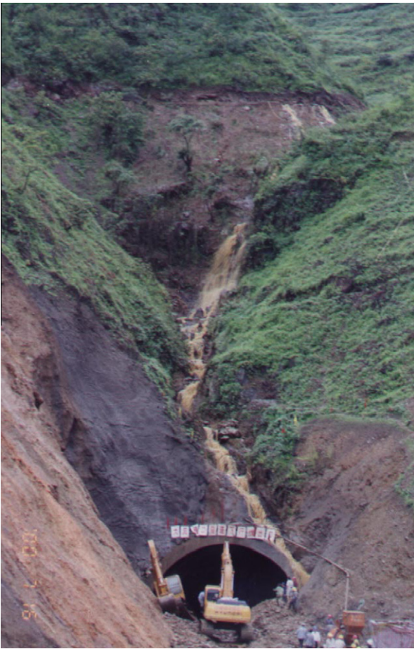
Fig. 3. The surface water near the valley flow to the tunnel portal.
